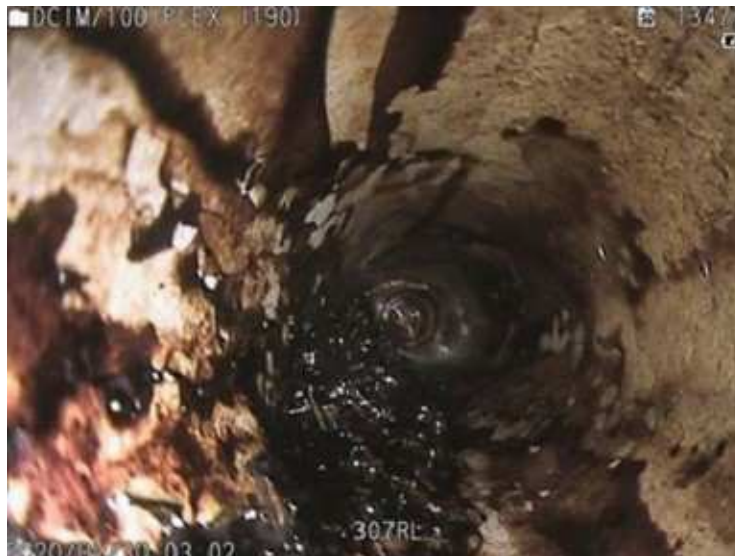
ONE-SIDED HEAVY COKE BUILD-UP EXAMPLES (NON-ACCEPTABLE CONDITION)
