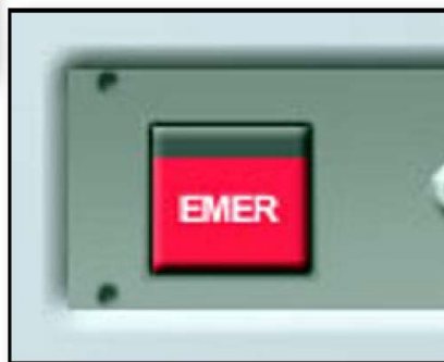
EMERGENCY LIGHTS - CONTROL AND INDICATING
