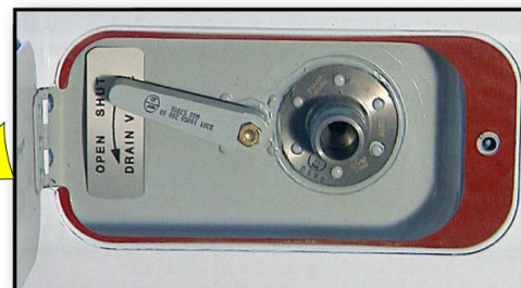
FWD DRAIN PANEL
