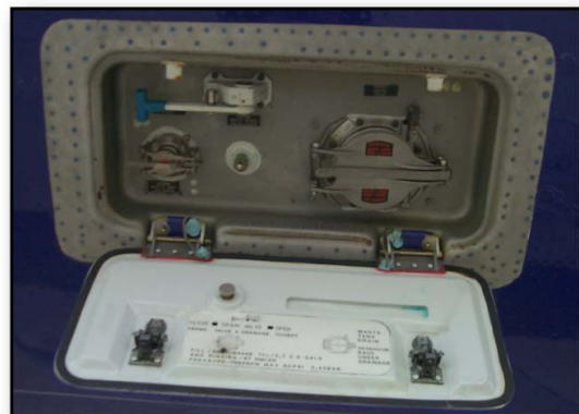
TOILET SERVICE PANEL
