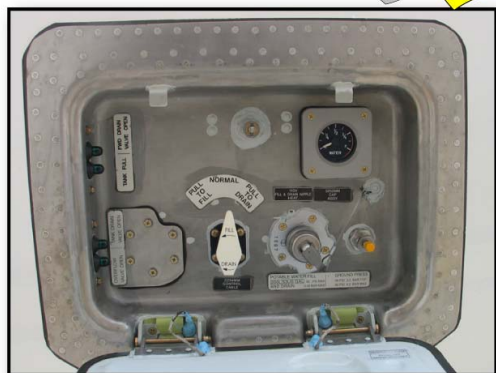
POTABLE WATER SERVICE PANEL
